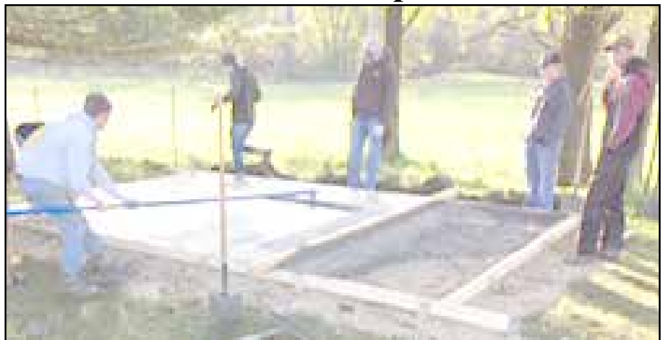
The weather cooperated Thursday for the Advanced Construction class to work at a job site north of Manchester and pour a 10' x 16' concrete slab. The next part of the project will be to build the shed, then transport and anchor it to the foundation.
